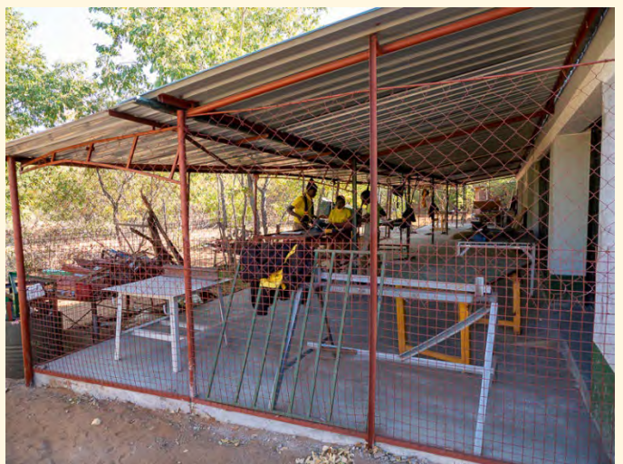
A recent extension to our Wood and Metal Tech classrooms to provide additional space
